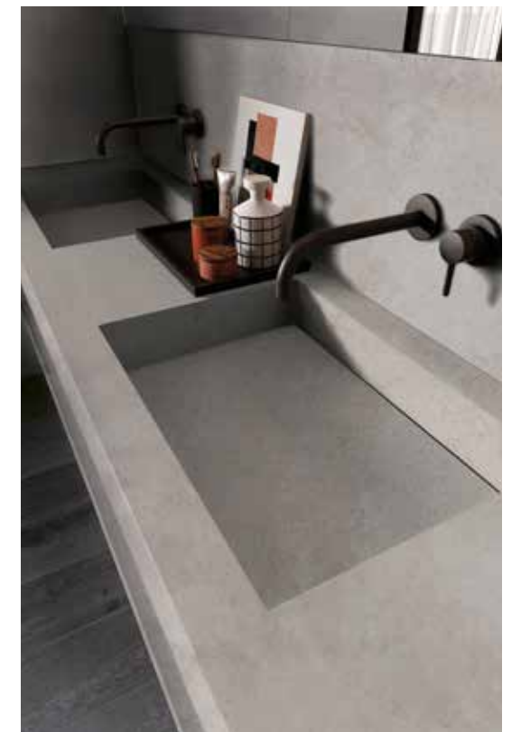
wall ALPES GREY integrated top with 2 washbasins and washbasin top ALPES GREY floor CROSSROAD WOOD COAL
